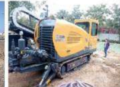
XZ360E水平定向钻机在河南郑州施工 XZ360E HDD works in Zhengzhou City, Henan Province
